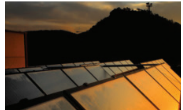
Solar power and geothermal energy contribute to the alternative energy portfolio of Magyar Posta
